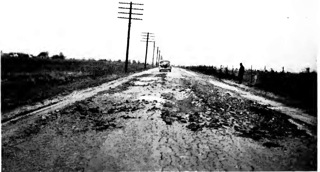
FROST DAMAGE—WINTER 1947-1948—ON U.S. ROUTE 213
